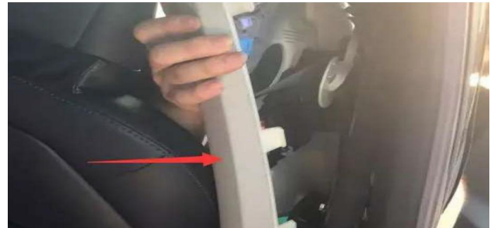
(12).拆下 B 柱上边饰板 用穿线绳将把手线从波纹管穿到车内，线材隐藏在车边沿饰板内 Remove the upper edge panel of pillar B and thread the handle line from the bellows to the inside of the car with the string, the wire is hidden in the edge panel of the car
