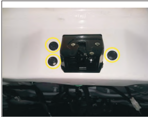
16. Remove the original car door lock, installed on our electric lock, use the original car screws
