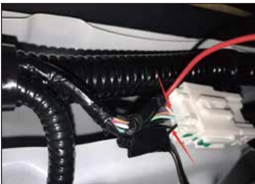
11. Front switch wiring mode, white and black color wires shown below docking method
