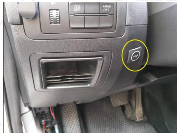
8. Remove the trim panel at the main driver, then punches a hole to install the front switch button.
